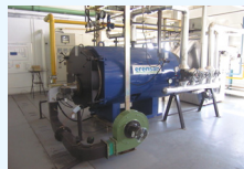
Boiler Training Unit
