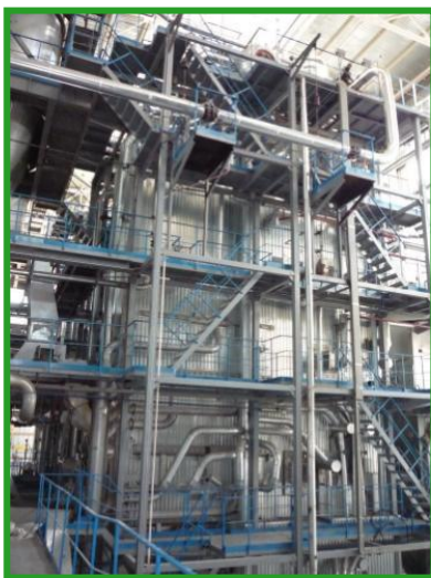
Steam boiler E-16-3,9-360 D
