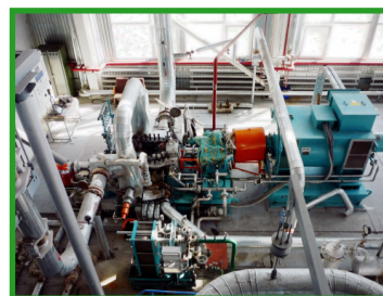
Steam turbine PBS Velkobites (Czech Republic)
