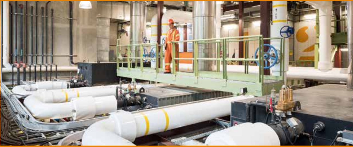
SEFC NEU Energy Centre
